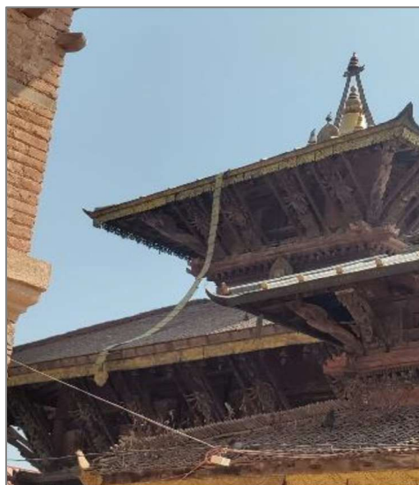
Figure 2. Changu Narayan temple located atop a small hill at Bhaktapur. The photograph depicts the down conductor dangling towards the bottom edge of the roof.
