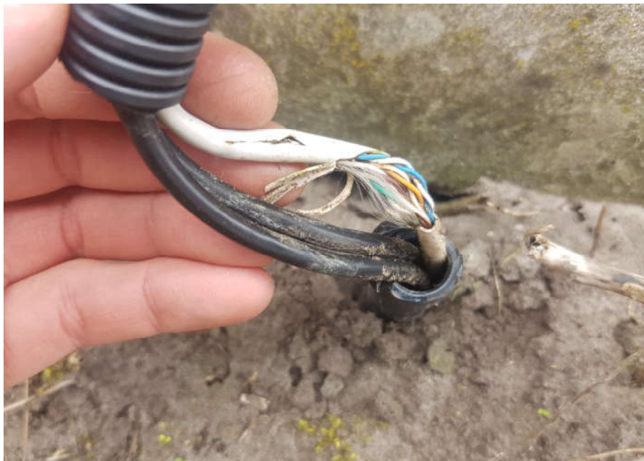
Figure 2 Cable interconnecting the antenna and the acquisition unit, two coaxial cables are used to transmit the analog signals from the antenna, the UTP cable secures the power for the integrated preamplifier and gain control.
